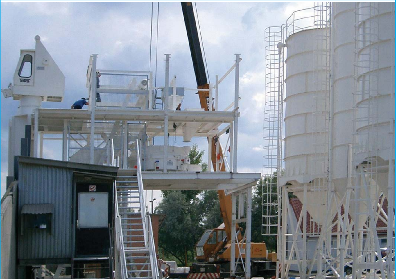
Montage MIXOMAT THZ 1500 B - S 5 Sternanlage • Erection MIXOMAT THZ 1500 B - S 5 scraper system
