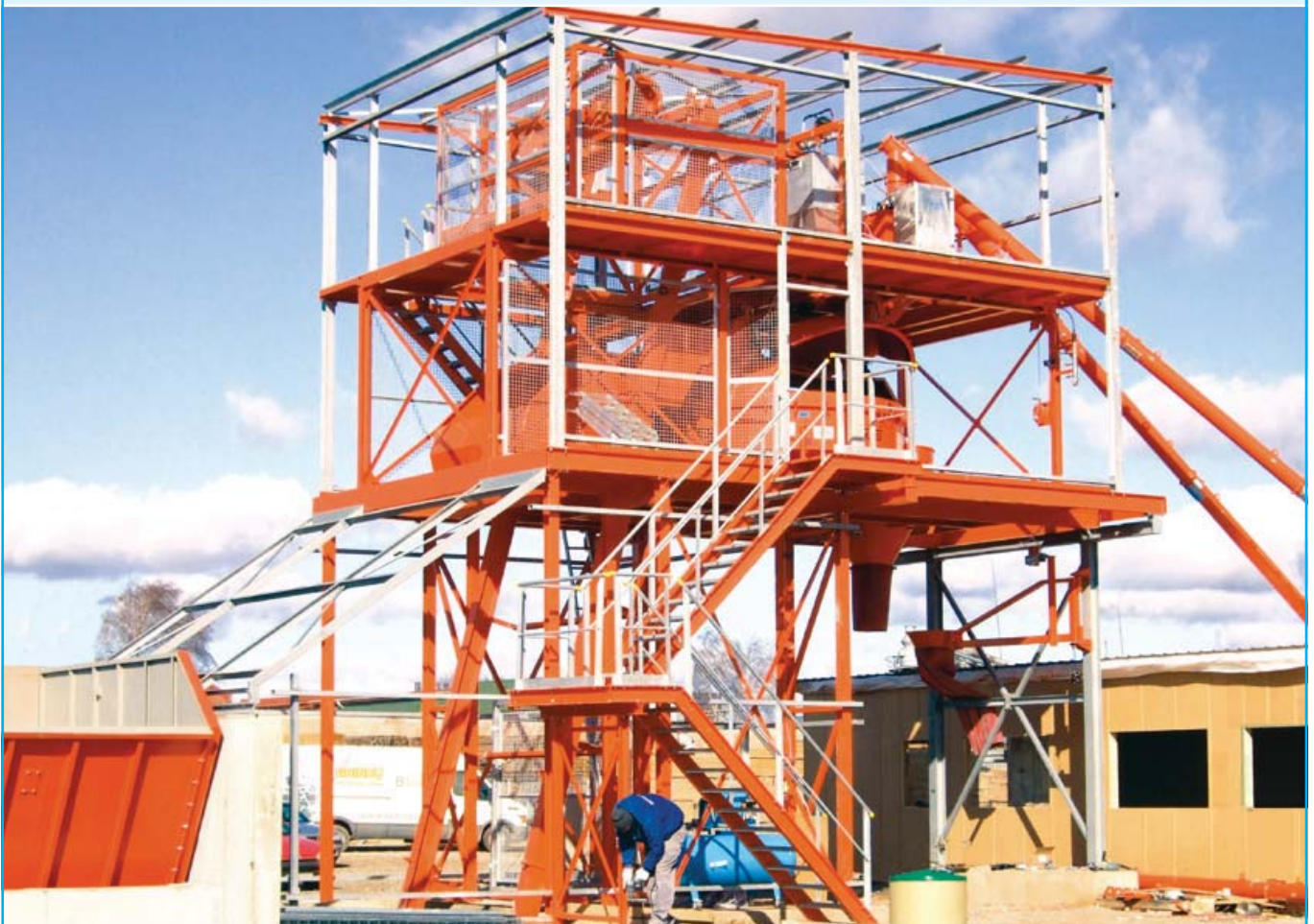
Montage MIXOMAT THZ 3000 - R 4 / 4 Reihen-Siloanlage, 4 Kammern • Erection MIXOMAT THZ 3000 B - R 4 / 4 aggregate in-line silo system, 4 compartments
